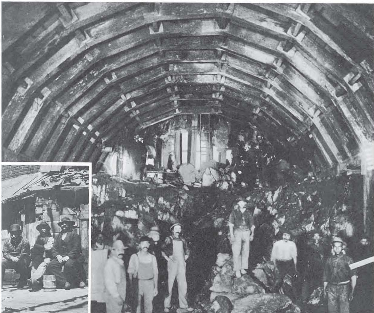
Construction of the Fort George IRT Tunnel, 1904. Courtesy of the New-York Historical Society, New York City
